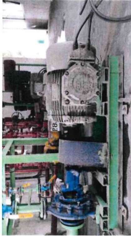
Photo -2 (Double Earthing pump)
